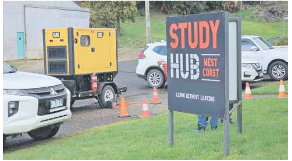
Emergency generator set up at the Zeehan Study Hub by the West Coast Council
